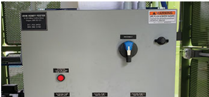
Splash Pad Control Unit
